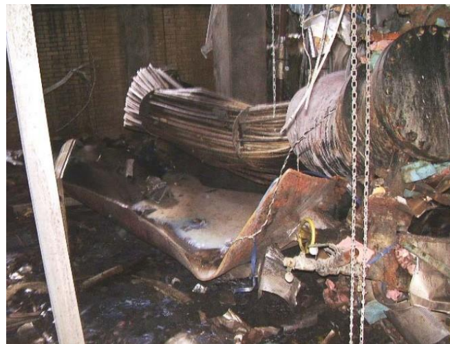
Figure 2: The remains of the ammonia heat exchanger, post-incident
