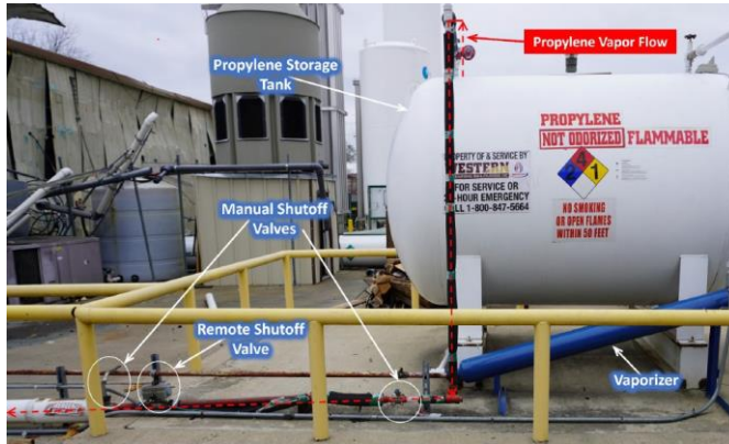
Figure 1: Post-incident photo of the propylene storage tank
